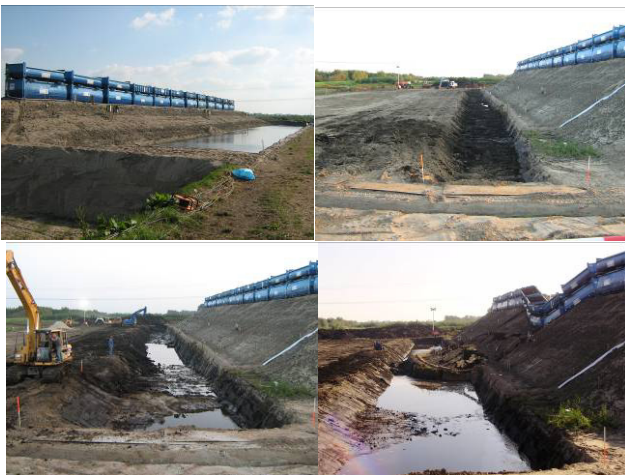
Figure 8. a) River side of the dike, b) Inner side of the dike during excavation of the ditch, c) Inner side of the dike after excavation of the ditch, d) Failure
